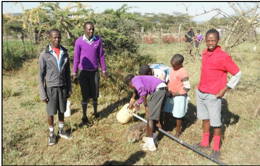
Masai children at the Nkenijii School near Narok, Kenya were able to get fresh water for the first time, thanks to a project by the Maywood, NJ Rotary Club that built a pipeline to the school from a spring 2-1/2 km away - with the help of WASRAG.
